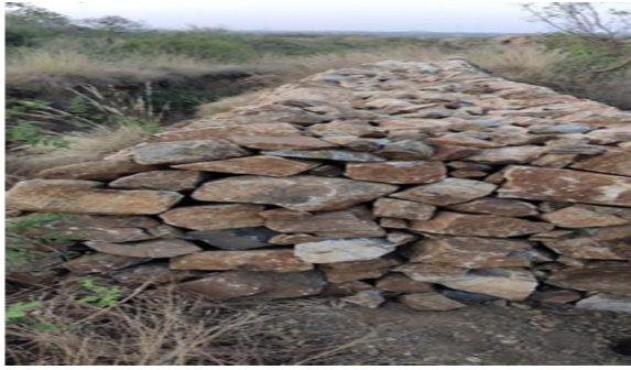
Rubble stone wall reinforcing damaged EPT
